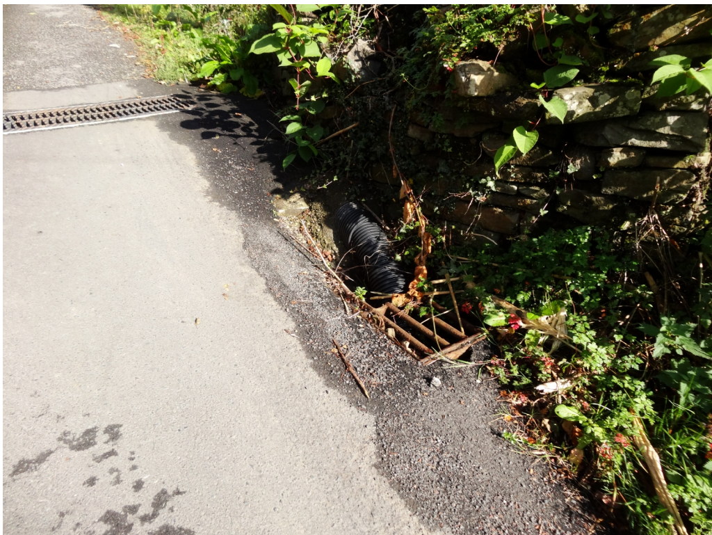
Plate 8: Plastic piping and recent scars on Graig-y-Merched roadway indicate ongoing movement and repairs.
